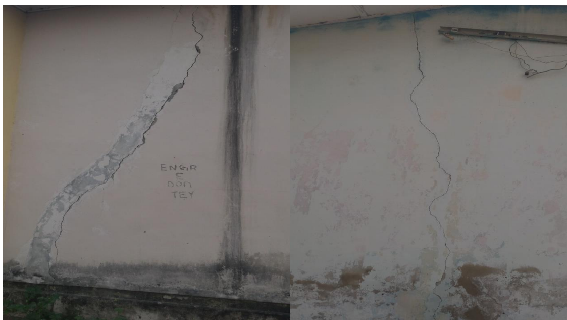
Plate 1: Section of the Cracks Wall in the Study Area
