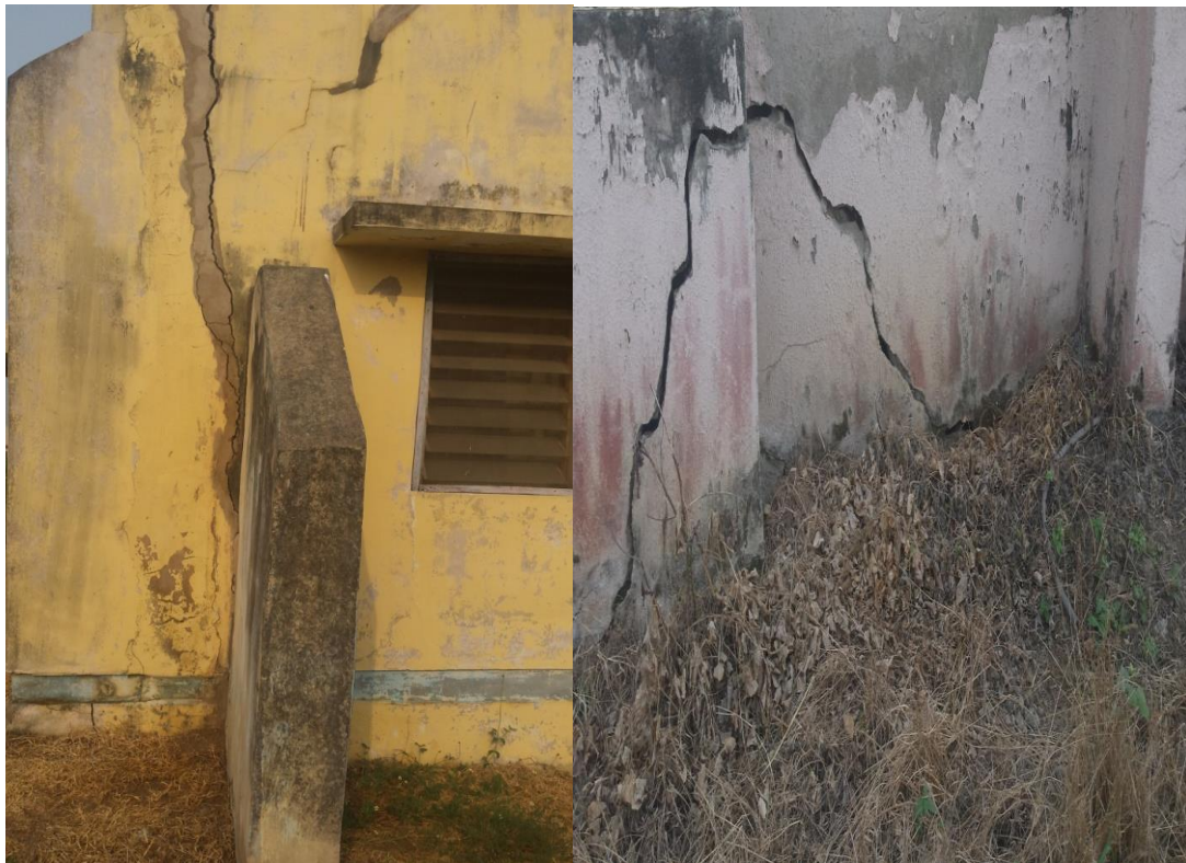
Plate 2: Section of the Cracks Wall in the Study Area
