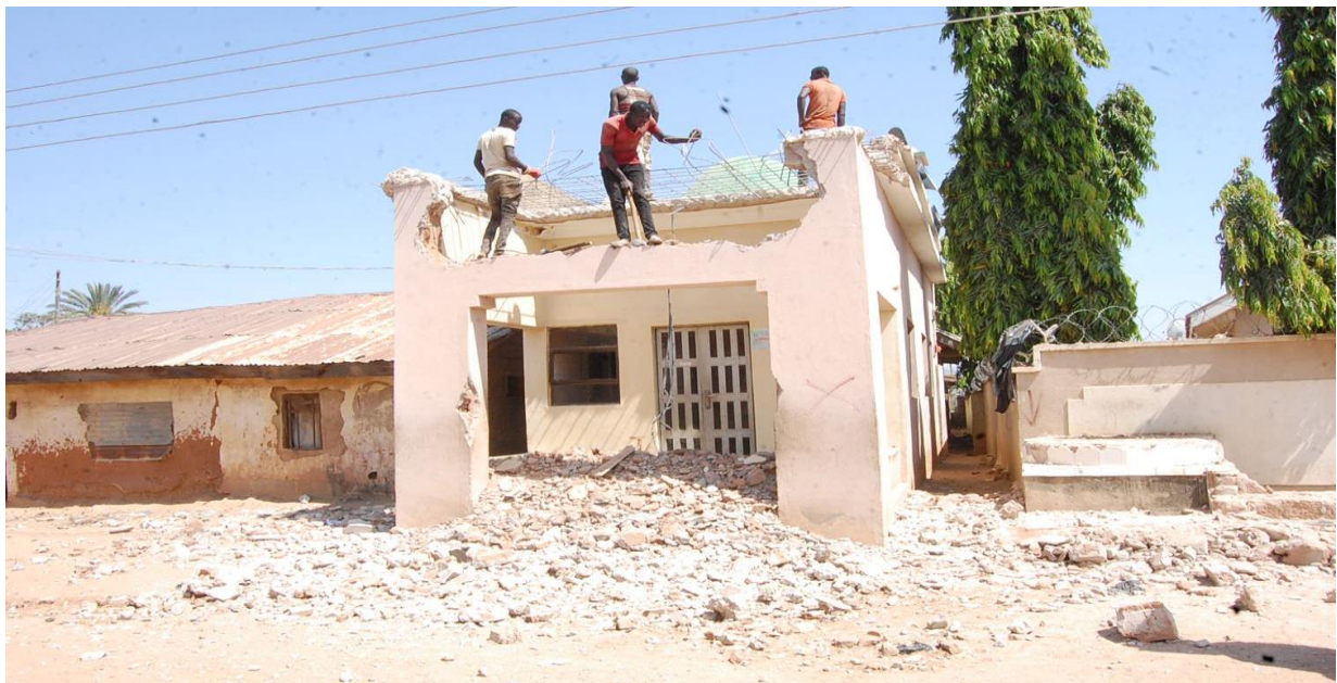
Plate 1: Demolition being carried out showing concrete debris on kasuwan doya road 4 in Lot 1
