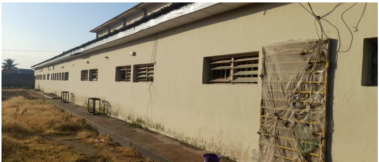
Plate 1: Sani Abacha Gymnasium in Bauchi is poorly lighted and ventilated.
