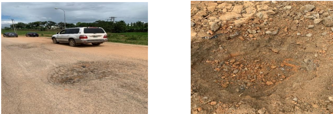
Figure 2.0: Showing Crack Types Damaged and Their Sample
