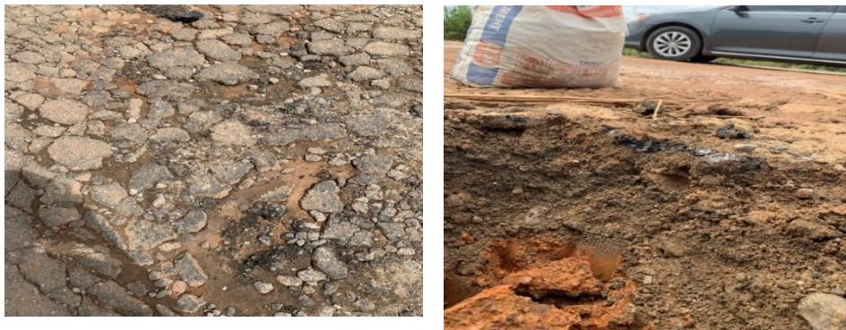
Figure 2.2: Showing of Distress Damaged and Their Sample
