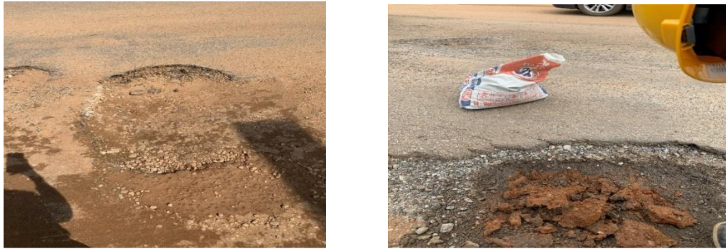
Figure 2.1: Showing Potholes Type Damaged and Their Sample
