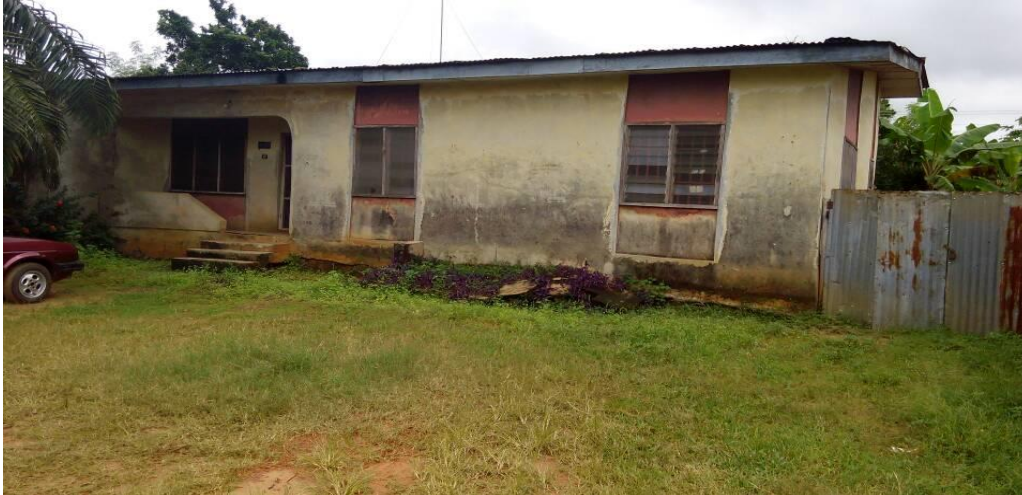
Plate 1: Photographic Image of the Semi-detached 3- Bedroom Bungalow at AHOCOL Phase 1 (AHOCOL 1) showing its appearance as a full-provision house rather than a partial-provision type (core house).
